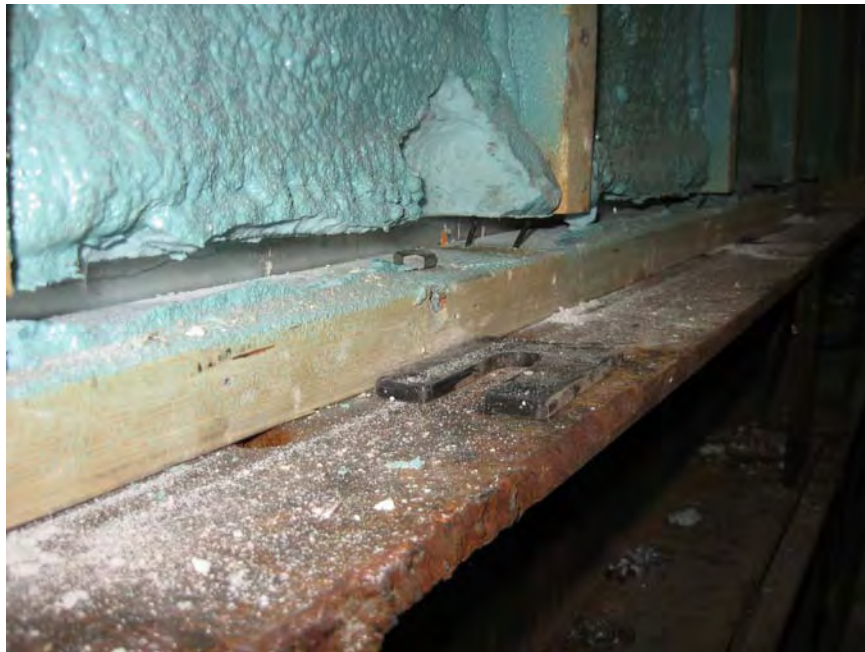
Photo No. 4 Sample #3 Stud Disengagement
